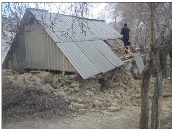
Destroyed house in Vanj | Red Crescent Society of Tajikistan
